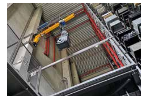
View of the stock shapes warehouse. The new drive motor hangs from a wall crane.
